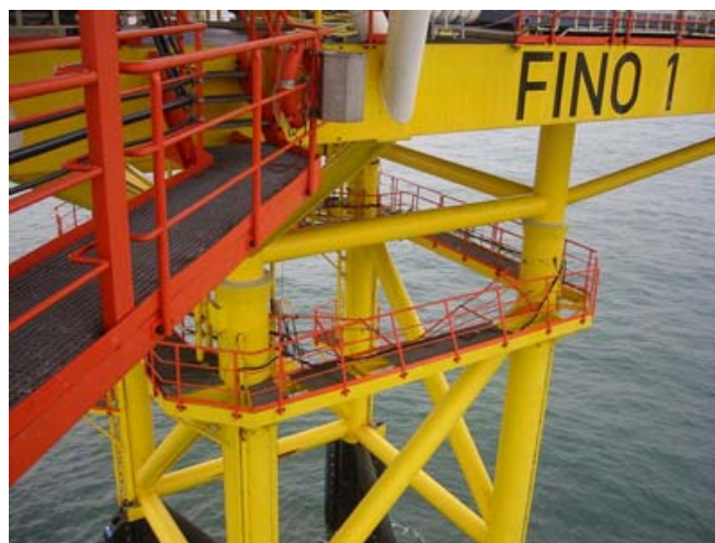
Fig. 4 Picture of the FINO platform showing the damage due to wave impact (BSH)
